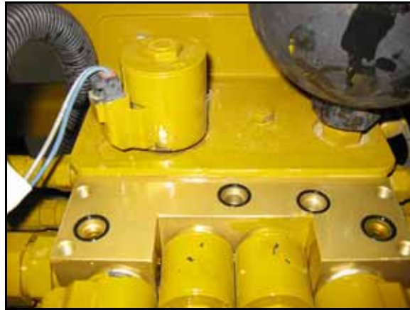
FIGURE 2. O-Rings Installed on the Machine's Hydraulic Valve
