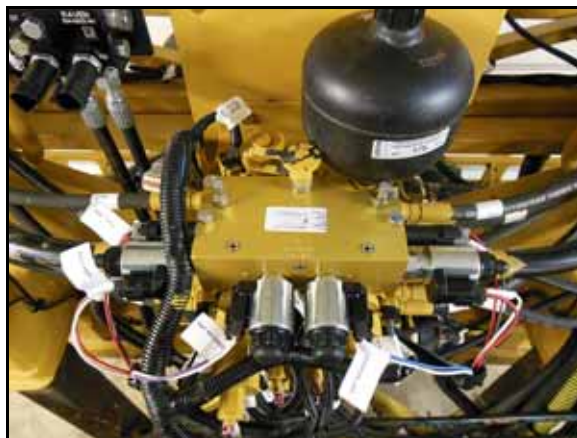
FIGURE 11. Valve Harness Installed on the AutoBoom Valve
