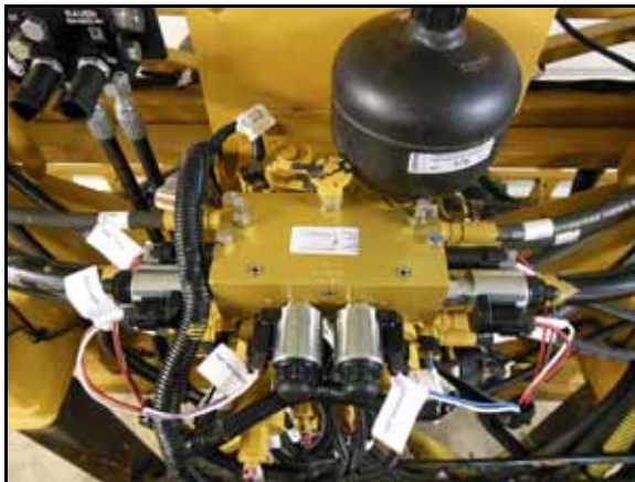
FIGURE 15. Valve Harness Installed on the AutoBoom Valve
