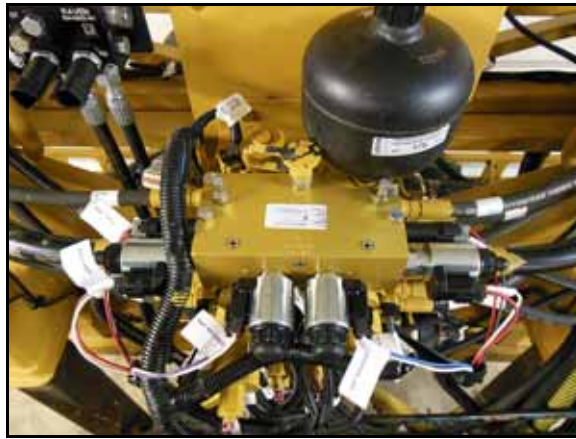
FIGURE 15. Valve Harness Installed on the AutoBoom Valve
