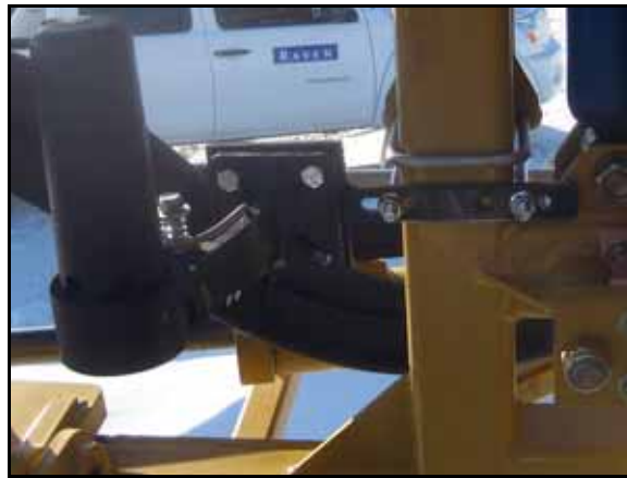
FIGURE 6. Center Rack Sensor Installed
