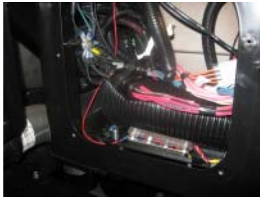
Connect to clean power buss bar.
