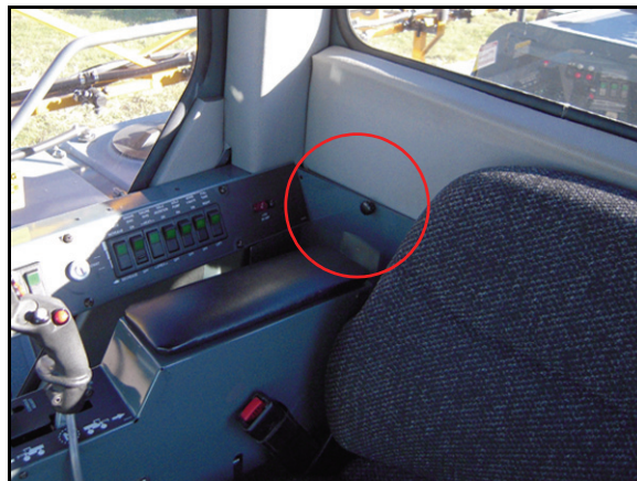
FIGURE 7. Machine's Electrical Distribution Panel
