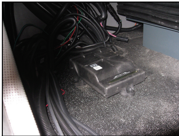
FIGURE 5. Node Mounted to Cab Floor
