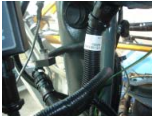
Tee into SCS 4600 Console Cable
