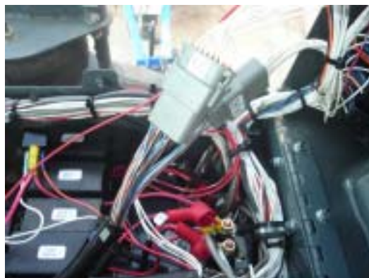
Tee into boom switch harness
