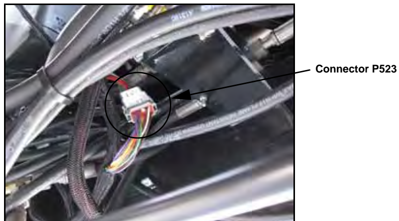
FIGURE 6. Fence Row Nozzle Connection
