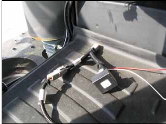
FIGURE 3. Power Tee Cable Connections
