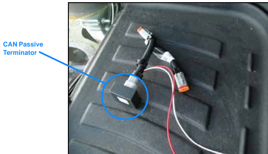
FIGURE 2. Power Tee Cable with Passive Terminator (P/N 063-0172-369) Installed
