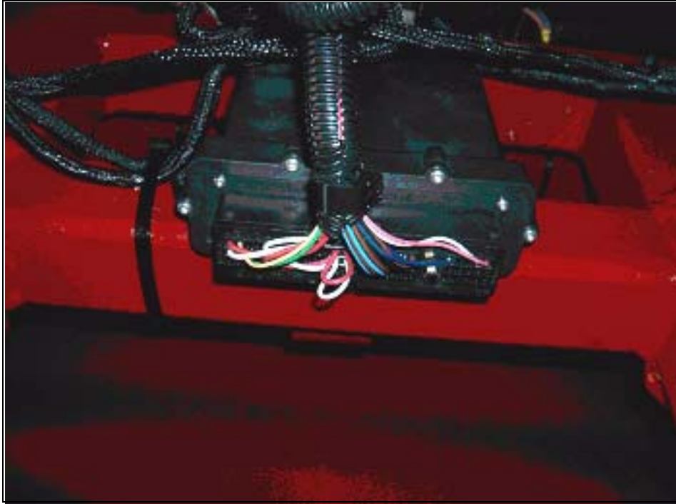
Accuboom cable connected to accuboom node.
