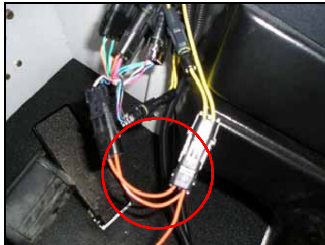
FIGURE 12. Master Boom Enable Switch Connected
