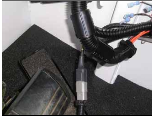
FIGURE 13. CAN Bus Cable Connected to the CAN Power Cable
