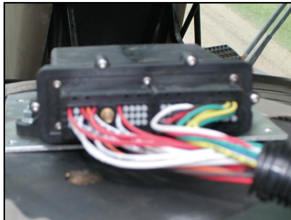
FIGURE 3. Raven Interface Cable Connected
