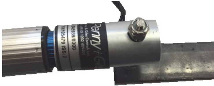
FIGURE 4. Old Sensor Installed
