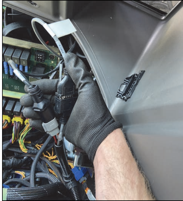
FIGURE 9. Smart Antenna Cable Connection
