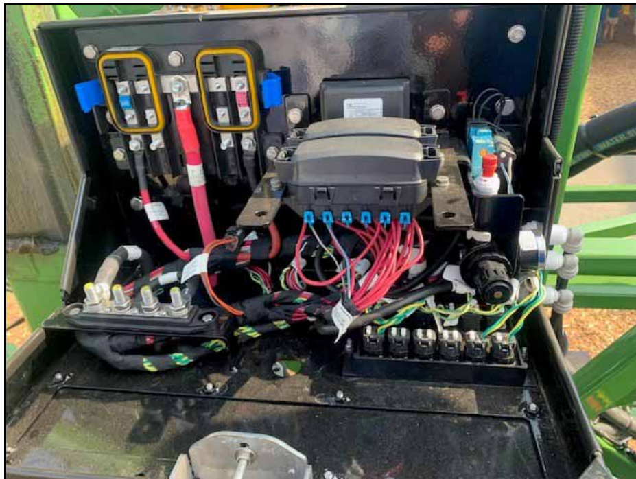
FIGURE 1. Power Distribution Cabinet without Hawkeye® 2 Installed
