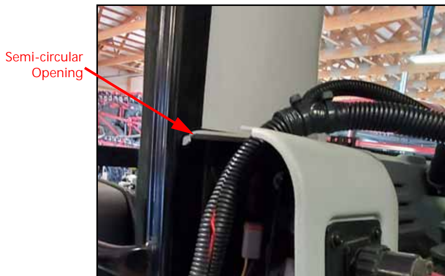
FIGURE 17. Power and Analog Video Cables Routed
