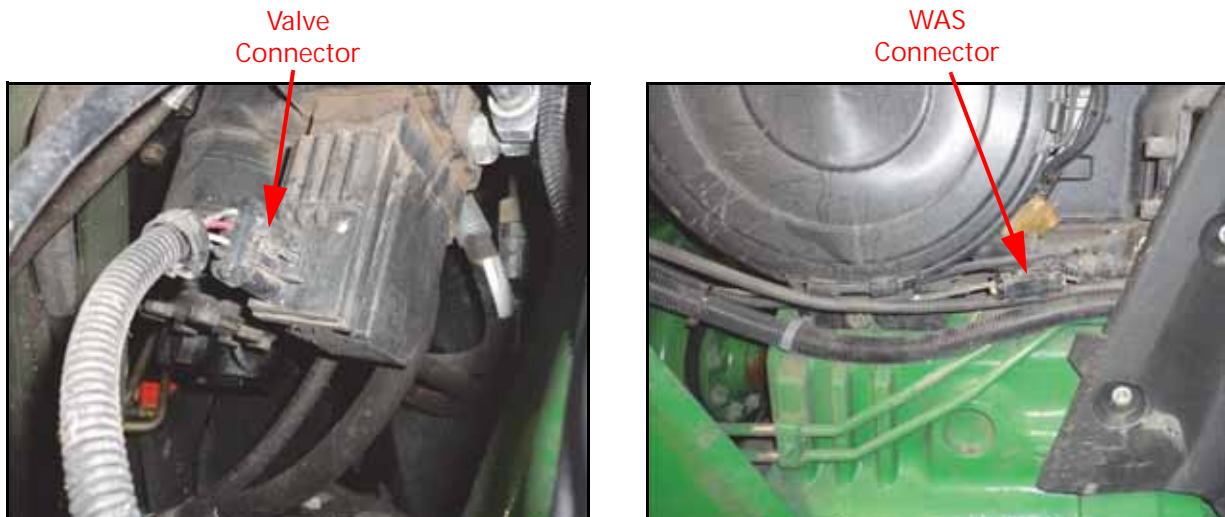
FIGURE 4. All Connected Cables
