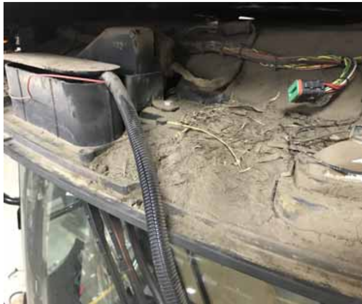
FIGURE 12. SC1 Receiver Cable
