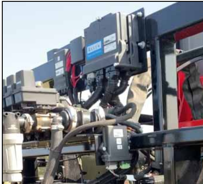
FIGURE 1. Electrical Panel Location
