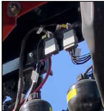
FIGURE 14. ET Apache Center Rack Ground Connection
