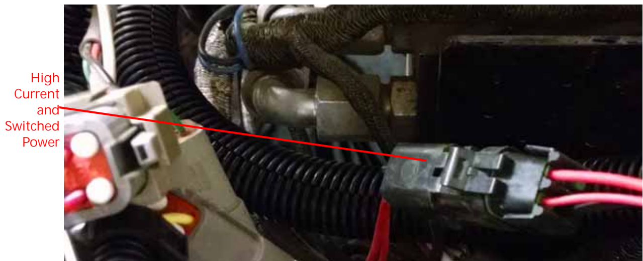
FIGURE 11. High Current and Switched Power Connection
