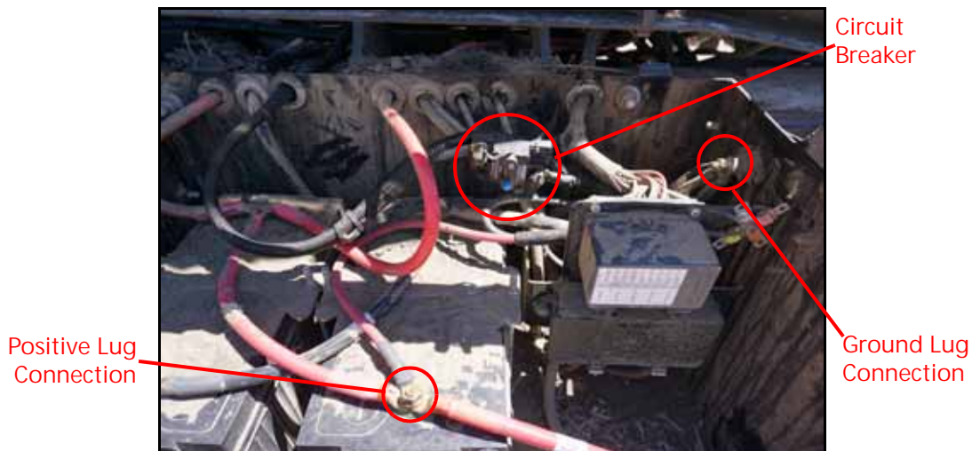
FIGURE 12. NCV2 High Current Power Battery Box Connections
