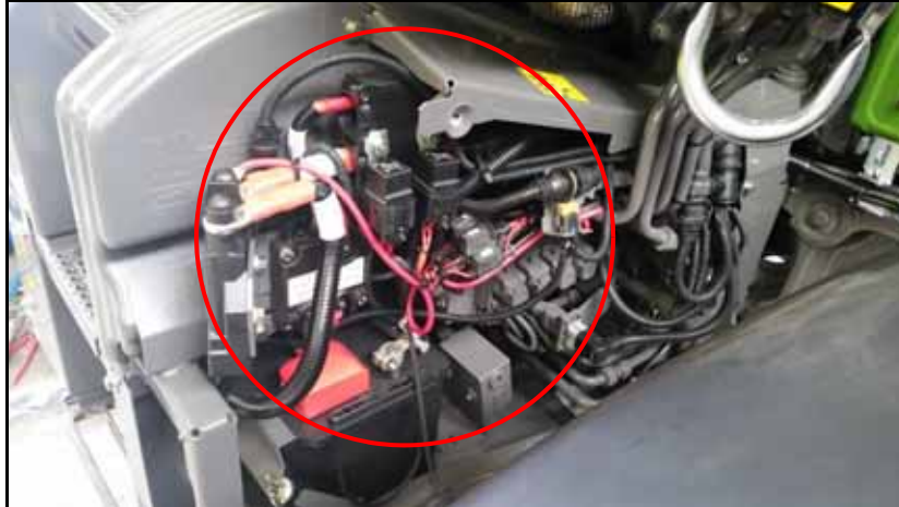
FIGURE 2. Relays and Fuses Correctly Mounted
