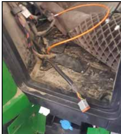
FIGURE 7. Cable Routed through Cab Floor
