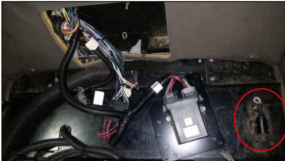
FIGURE 15. SC1 Node Mounting Location
