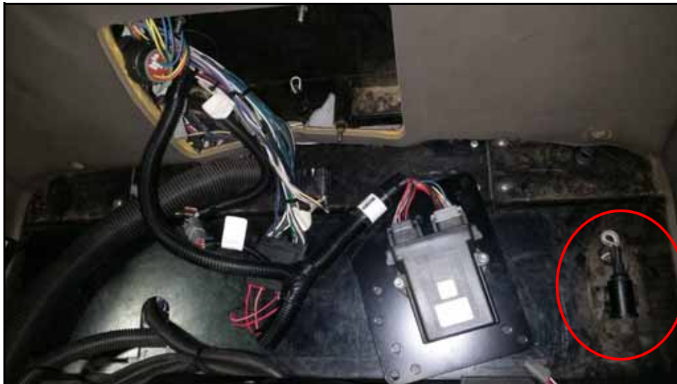
FIGURE 12. SC1 Node Mounting Location
