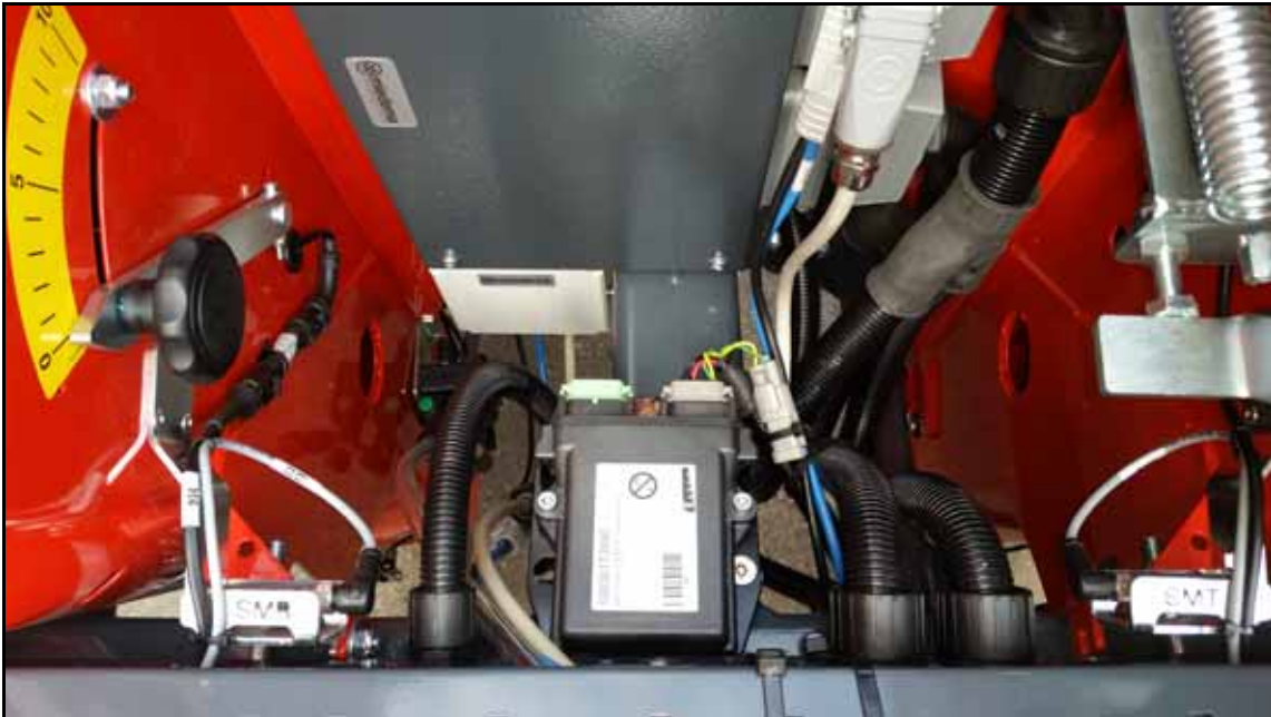
FIGURE 10. SC1 ECU Mounted
