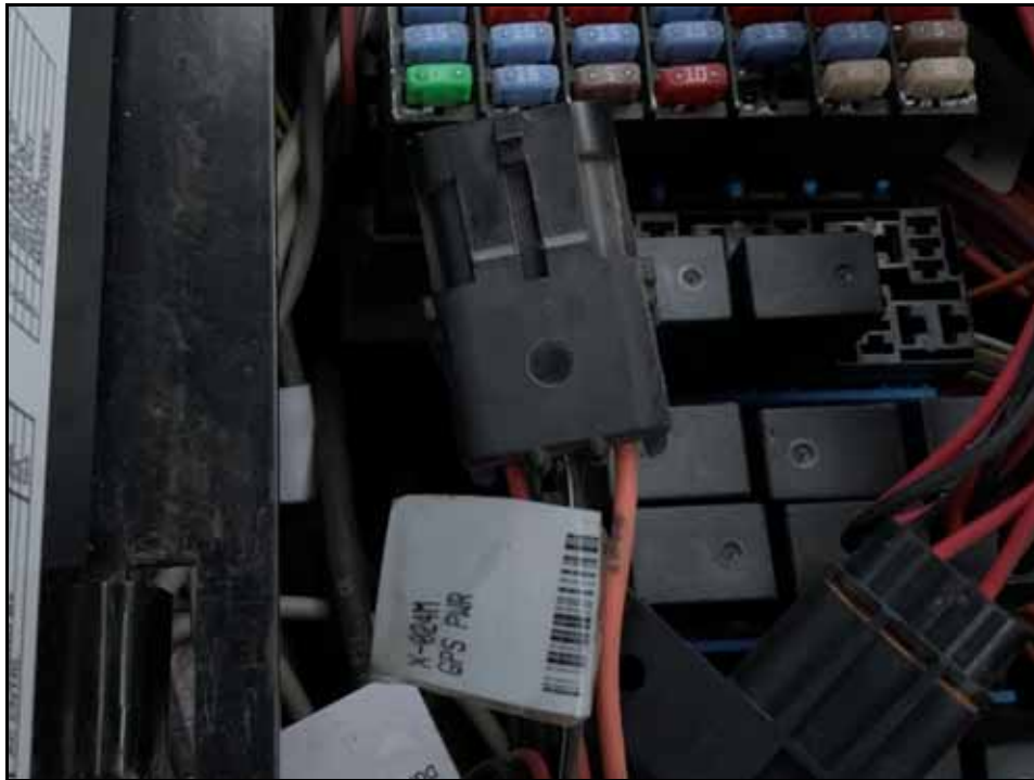
FIGURE 16. Existing Machine GPS Power Connector
