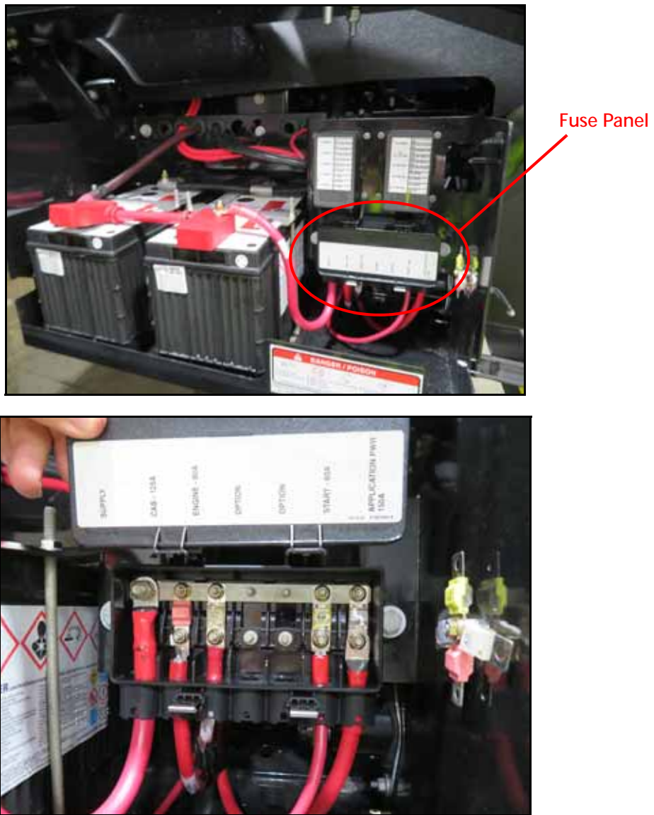
FIGURE 12. Fuse Panel Location
