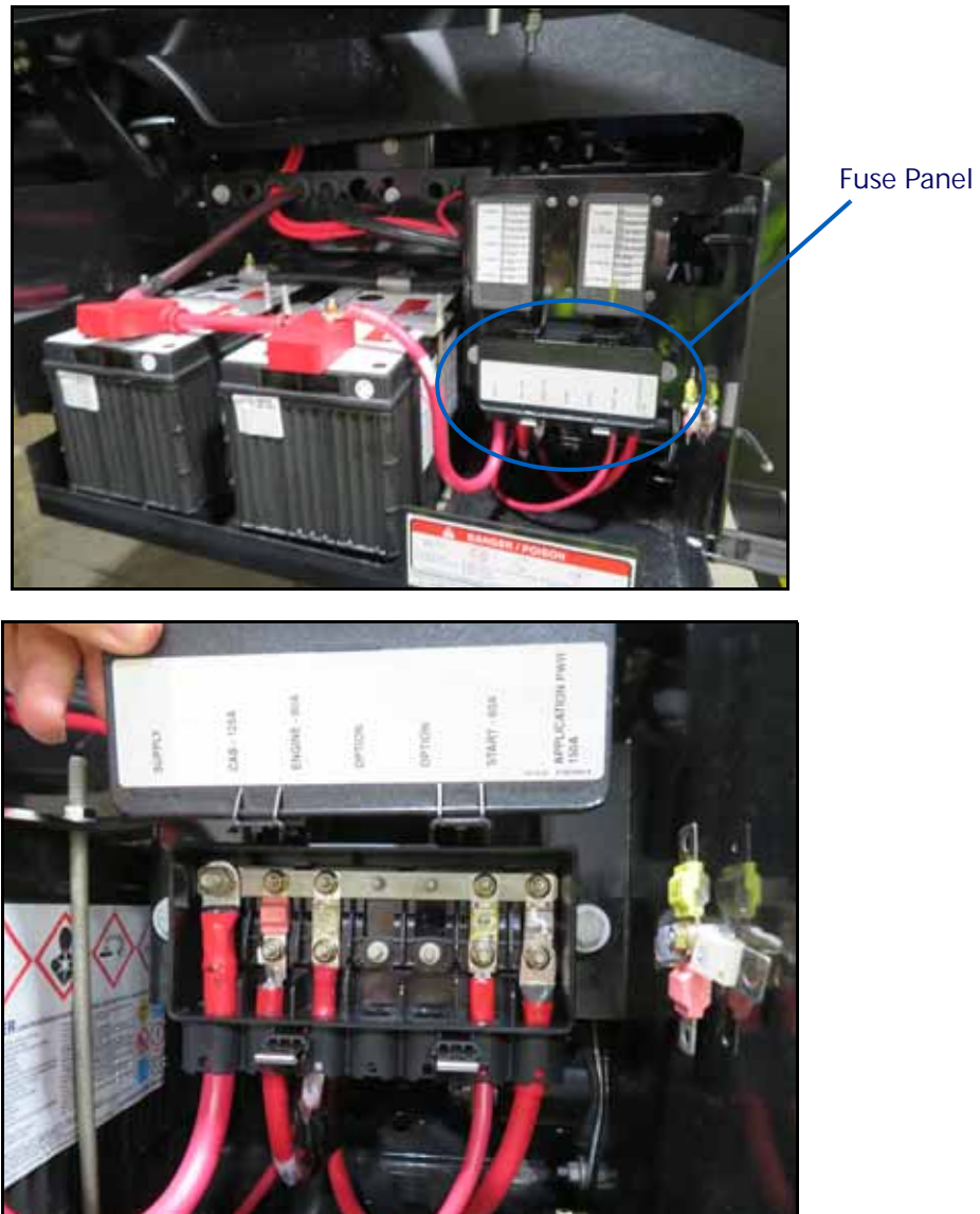
FIGURE 12. Fuse Panel Location
