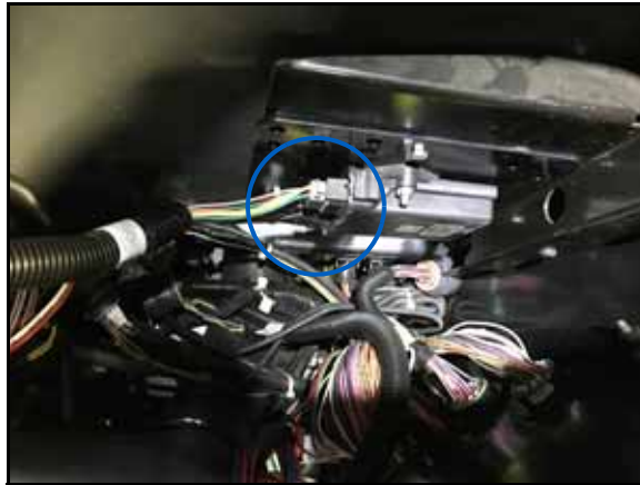
FIGURE 9. HDU Harness Connectors Connected to HDU
