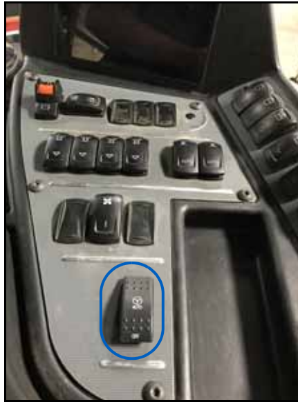
FIGURE 15. Steering Lockout Switch Installed
