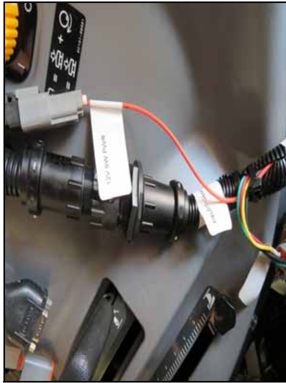
FIGURE 11. Switched Power and Field Computer Connections
