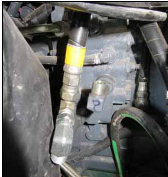
FIGURE 16. BSPP Elbow Connected to Tank Tee Port
