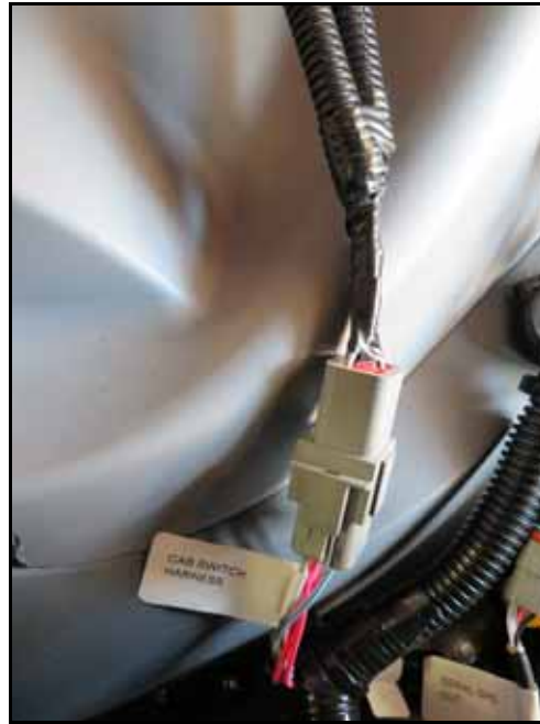
FIGURE 12. Cab Switch Harness Connection
