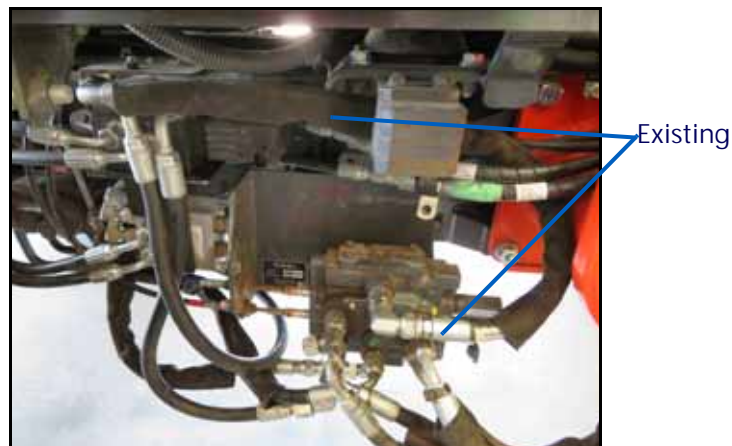
FIGURE 15. Existing Pressure Hose Connected to Steering Valve
