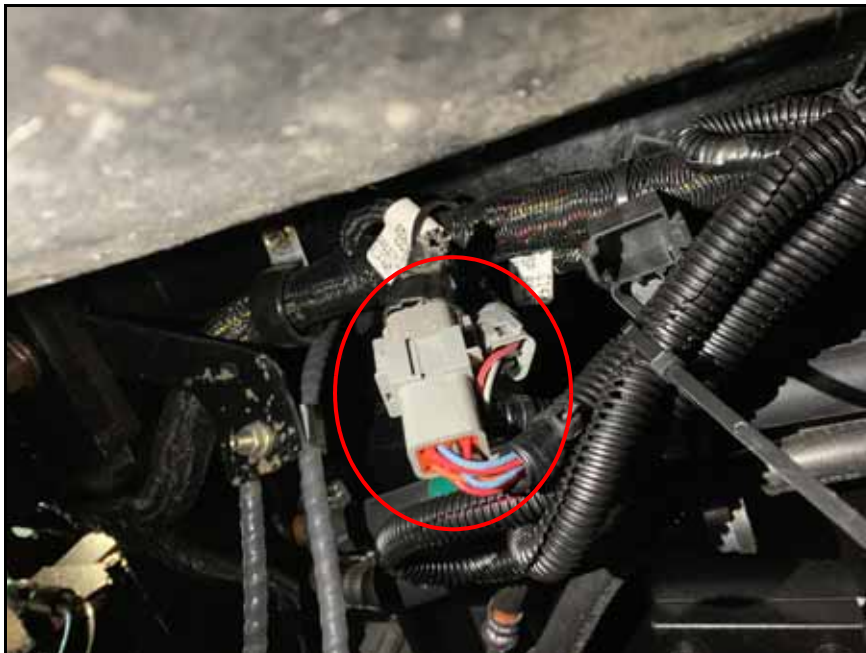
FIGURE 6. Valve Harness Connection
