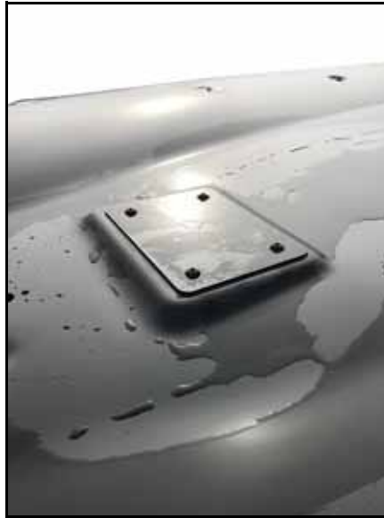
FIGURE 3. RS1 Mounting Location on Roof
