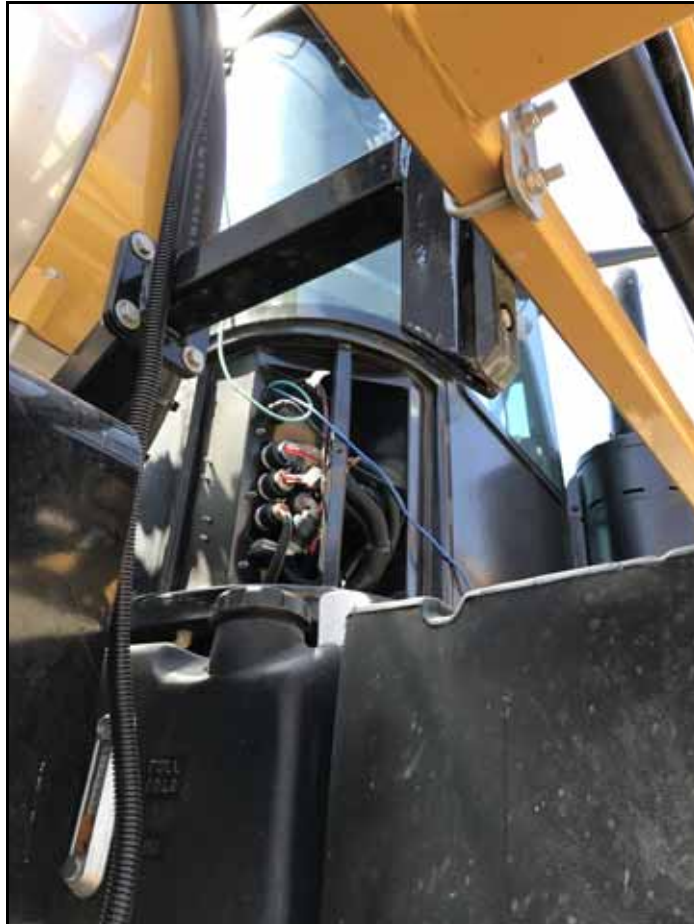
FIGURE 7. Exterior Cab Access Panel Removed from Right Rear
