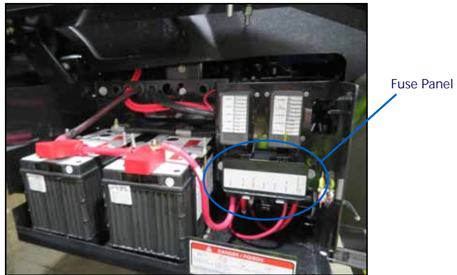
FIGURE 10. Fuse Panel Location
