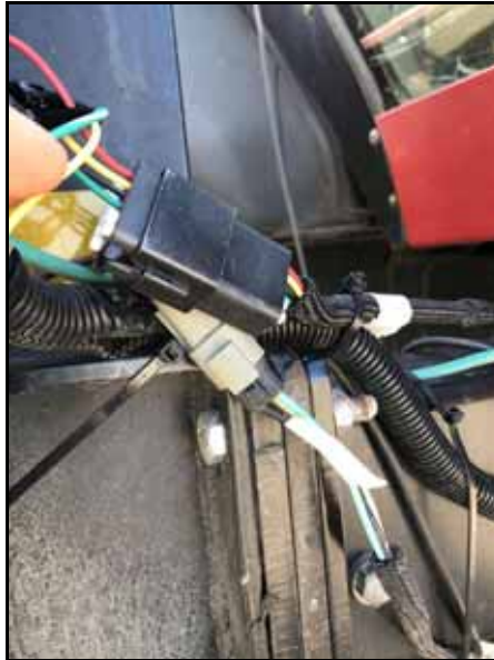
FIGURE 20. 12-Pin Aux Sensor Connected to VSN Cable
