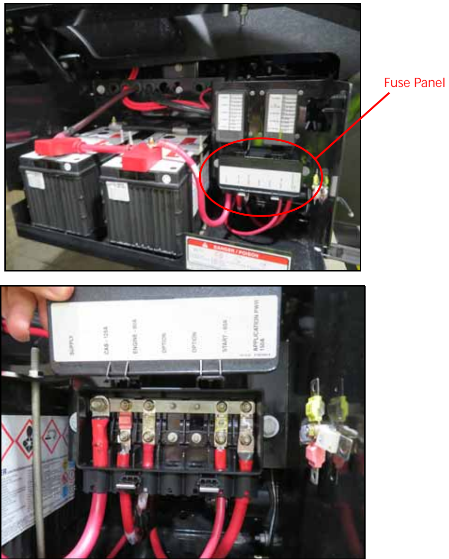
FIGURE 13. Fuse Panel Location
