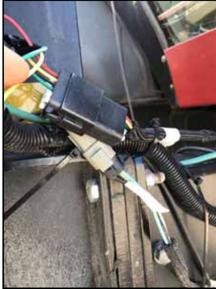
FIGURE 22. 12-Pin Aux Sensor Connected to VSN Cable
