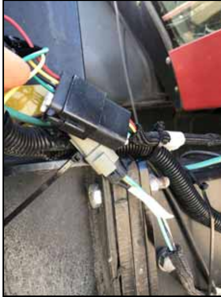
FIGURE 22. 12-Pin Aux Sensor Connected to VSN Cable
