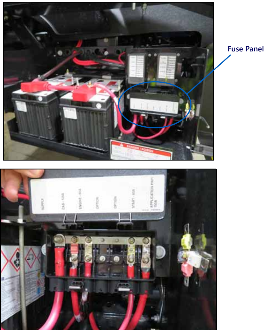
FIGURE 13. Fuse Panel Location
