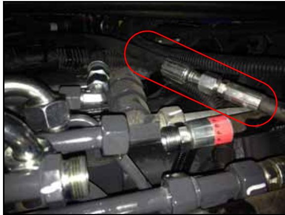
FIGURE 23. Hydraulic Hose Installed on Load Sense Hose
