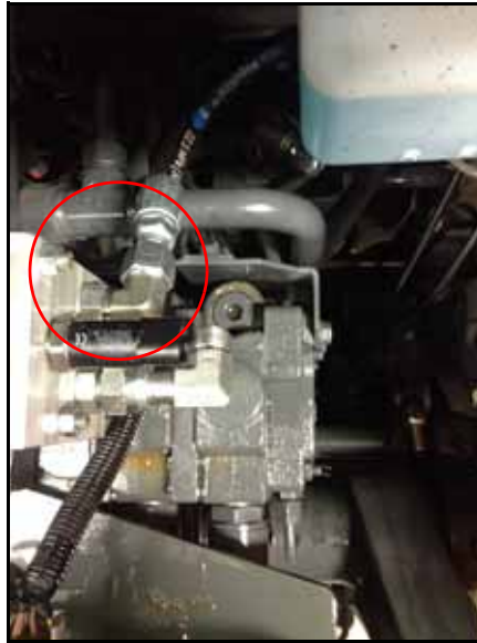
FIGURE 11. Hydraulic Hose Installed on Port A of the Dual POCI Valve
