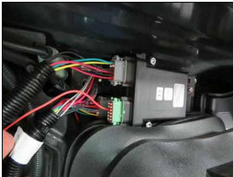
FIGURE 3. TC1/HDU Cable Connection
