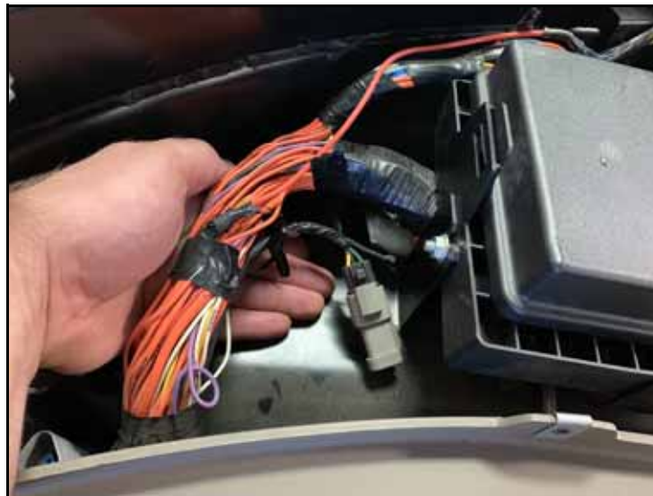
FIGURE 10. CAN Terminator inside Removed Cover
