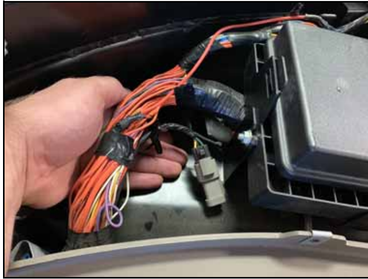
FIGURE 9. CAN Terminator inside Removed Cover
