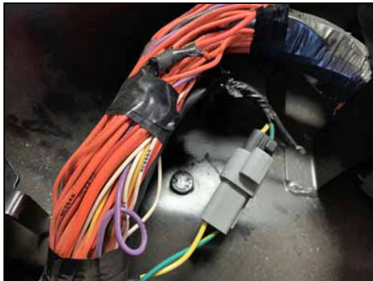
FIGURE 10. HDU Cable Connected to Machine Harness
