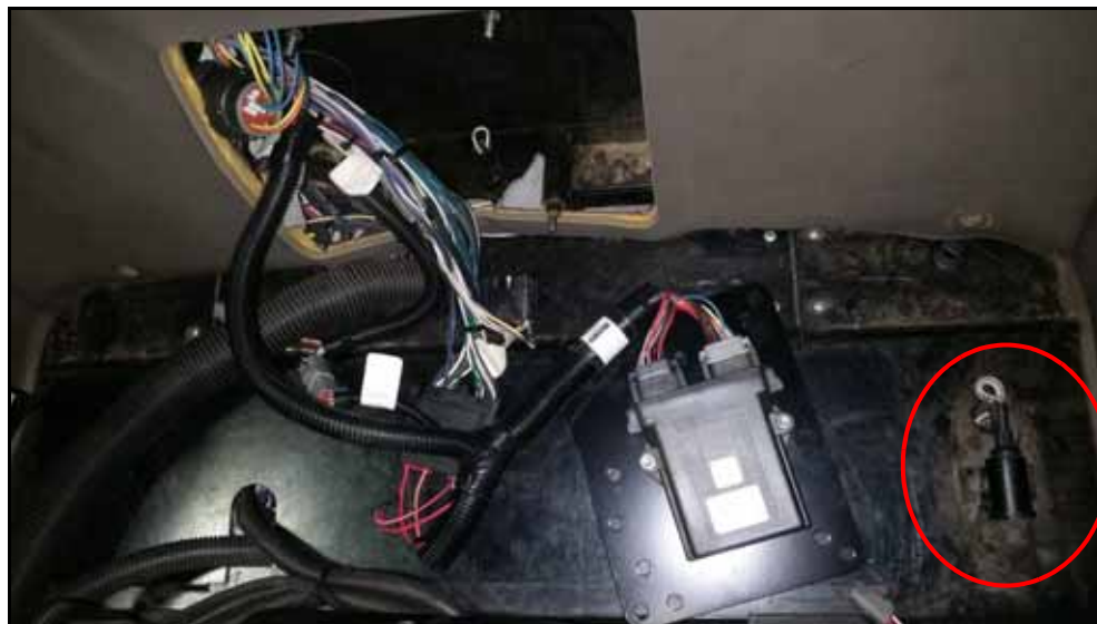
FIGURE 10. SC1 Node Mounting Location
