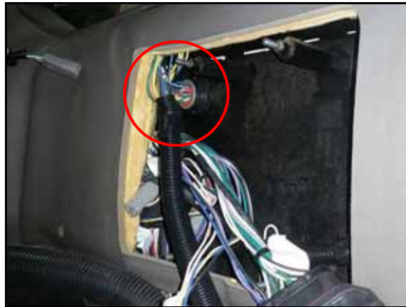
FIGURE 3. Machine's XB-7 Bulkhead Connection
