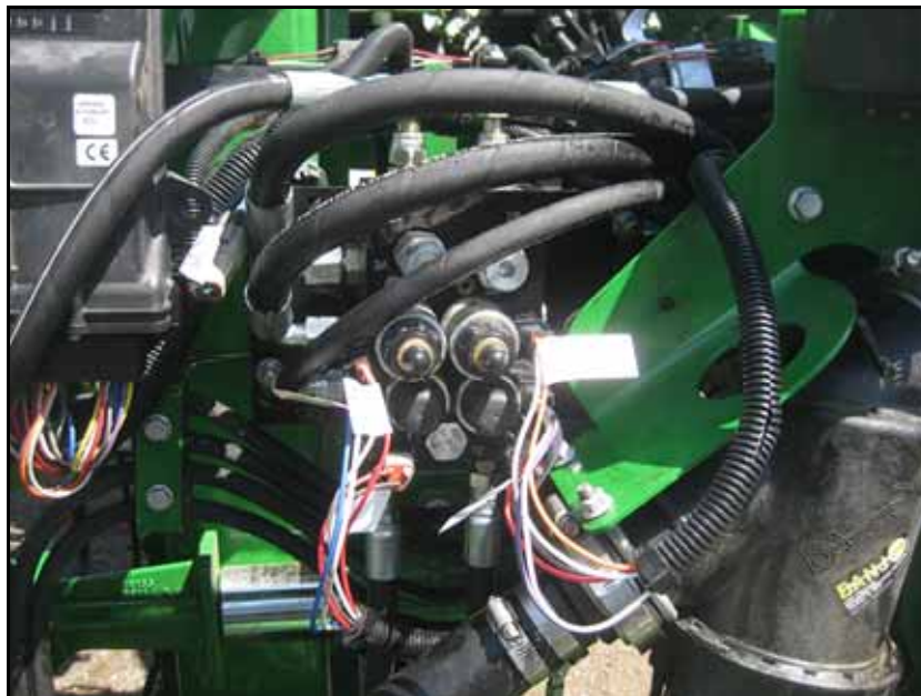
FIGURE 8. Electrical Connections on AutoBoom Valve
