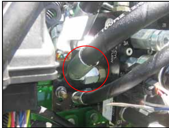
FIGURE 12. Pressure Hose Installed on AutoBoom Valve
