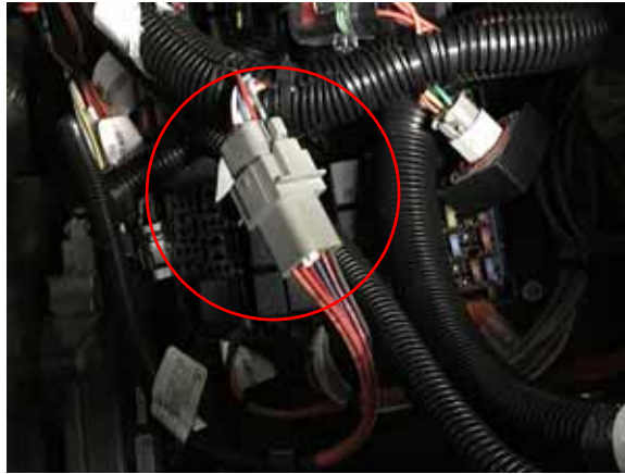
FIGURE 15. HDU Harness Cable Connection
