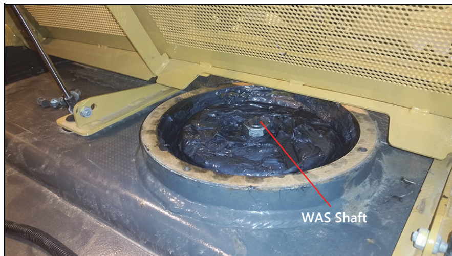
FIGURE 13. Installed WAS Shaft
