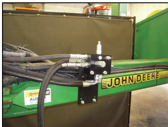
FIGURE 17. Pressure-Reducing Valve Pressure and Tank Hoses Installed
