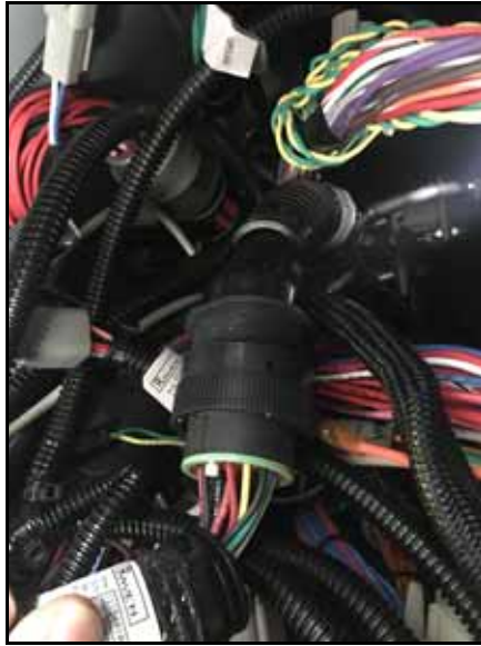
FIGURE 13. HDU Cable Connection in the Cab
