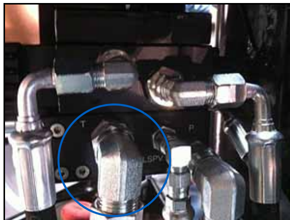
FIGURE 14. Tank Hose Installed on Steering Valve
