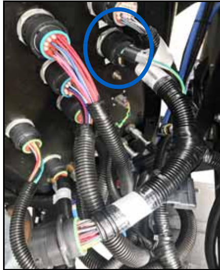
FIGURE 23. Bulkhead Connector to HDU Cable
