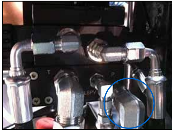
FIGURE 12. Pressure Hose Installed on Steering Valve
