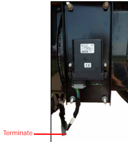
FIGURE 9. AutoBoom Cable Connected to Node
