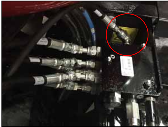
FIGURE 13. Load Sense Hose Installed on Valve
