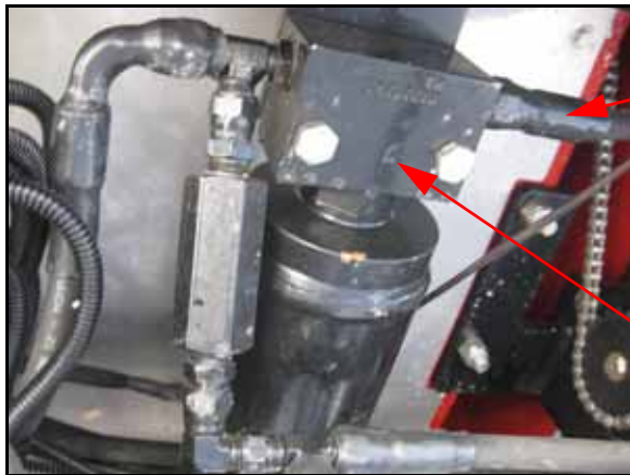
FIGURE 14. Machine's Right Accumulator
